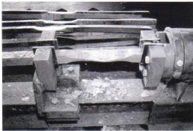
This twist can be done in a vise, but this manual twister helps keep the bar straight and speeds the process.
