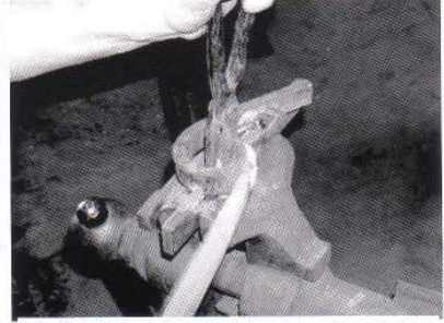
A scroll tool was made for this job. Scroll tongs clamp the pre-formed bar at the proper starting position.
