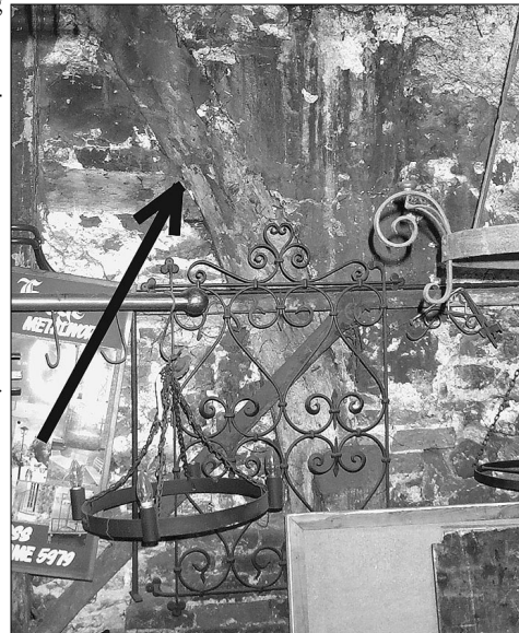
Arrow points to a curved structural beam embedded in the masonry of an original area of the building. Zeke told us that the Ancients often strapped young trees so as to force them to grow into the curved shapes desired for structural arches. The use of this technique diminished after the fifteenth century, leading the Moss’s to believe that this portion of the structure might possibly date to that period.
